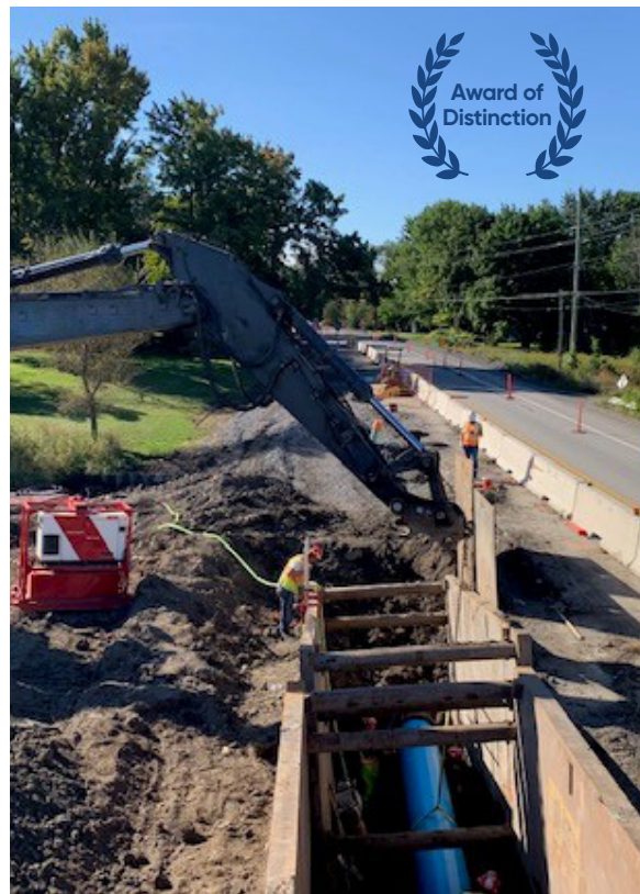
JL Richards won an Ontario Engineering Project Award of Distinction for this project.
