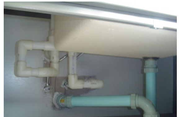
IPEX Enpure™ was used for high purity processing of water and reverse osmosis distribution system
