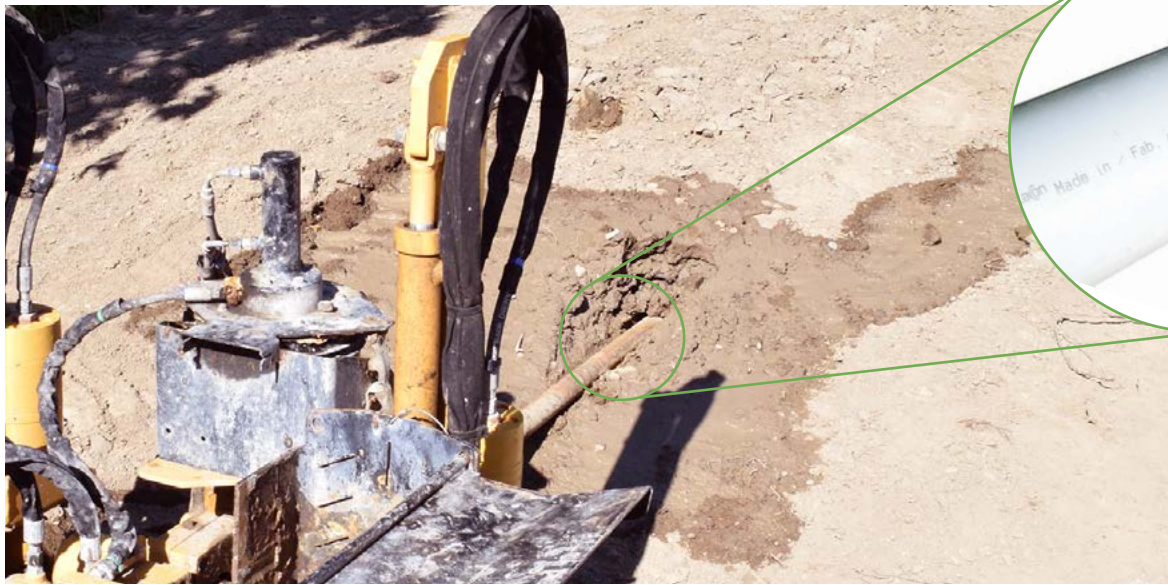
Two 60-foot lengths of SceptaCon raceway were installed while traffic still flowed
