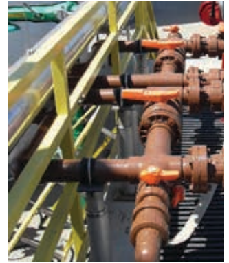
IPEX PVC & CPVC systems were painted brown with latex paint for chemical identification and UV protection.
